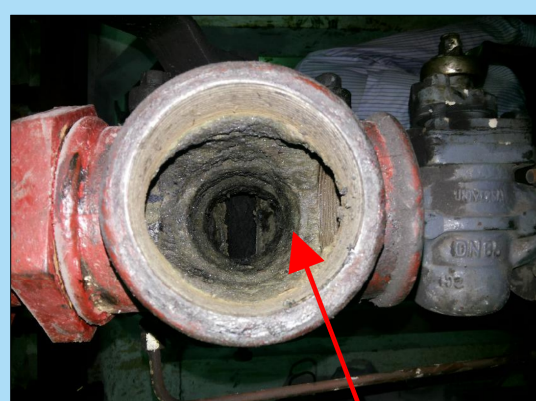
Naphthalene deposition in CO Gas Pipe line
